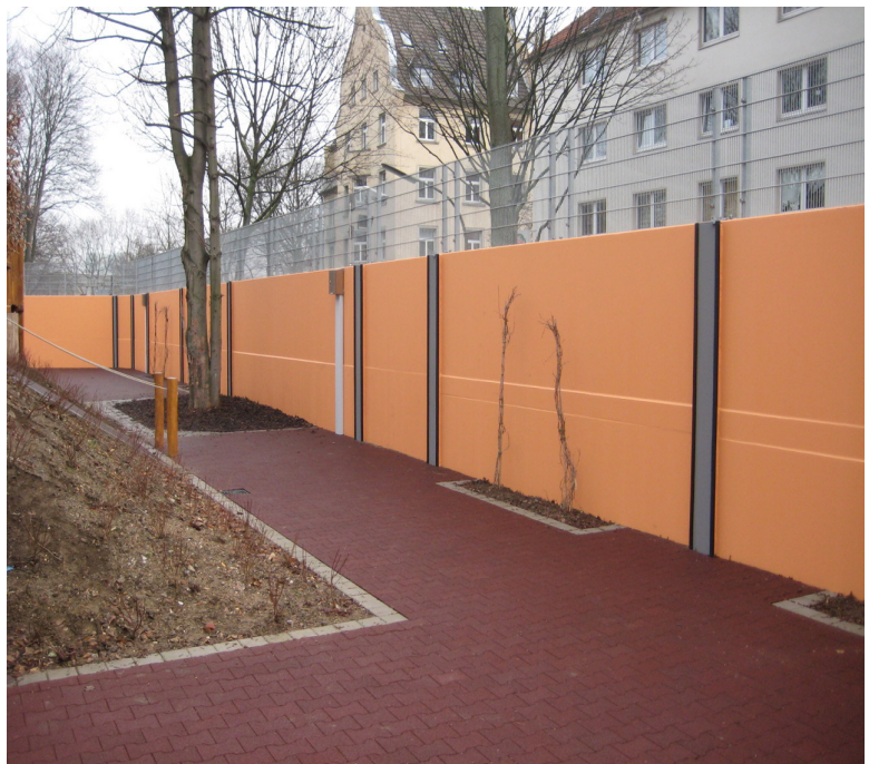
Protective wall endangered facility, Germany
