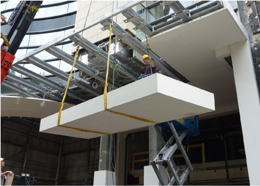
Fig. 16: Installation of ceiling panels with up-stands to cover the steel structure (l = 7,5 m, 25 ft / d = 70 mm, 2.8")
