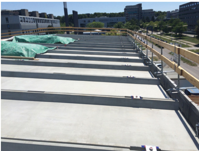
Fig. 34: Activated and load bearing roof panels (h = 10,6 m, 35 ft / l = 42 m, 140 ft)
